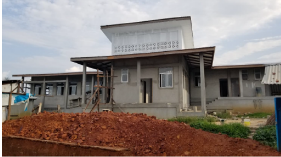
floor view, Current status as of June 9, 2021, painting works ongoing, septic tank construction ongoing in the foreground
