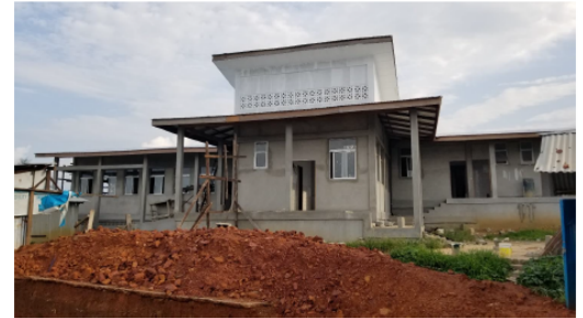
Rear view. Current status as of June 9, 2021, painting works ongoing, septic tank construction ongoing in the foreground
